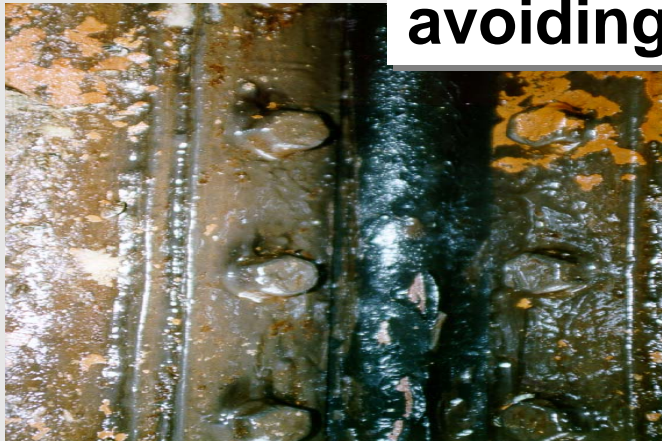
Failure of the joint material
